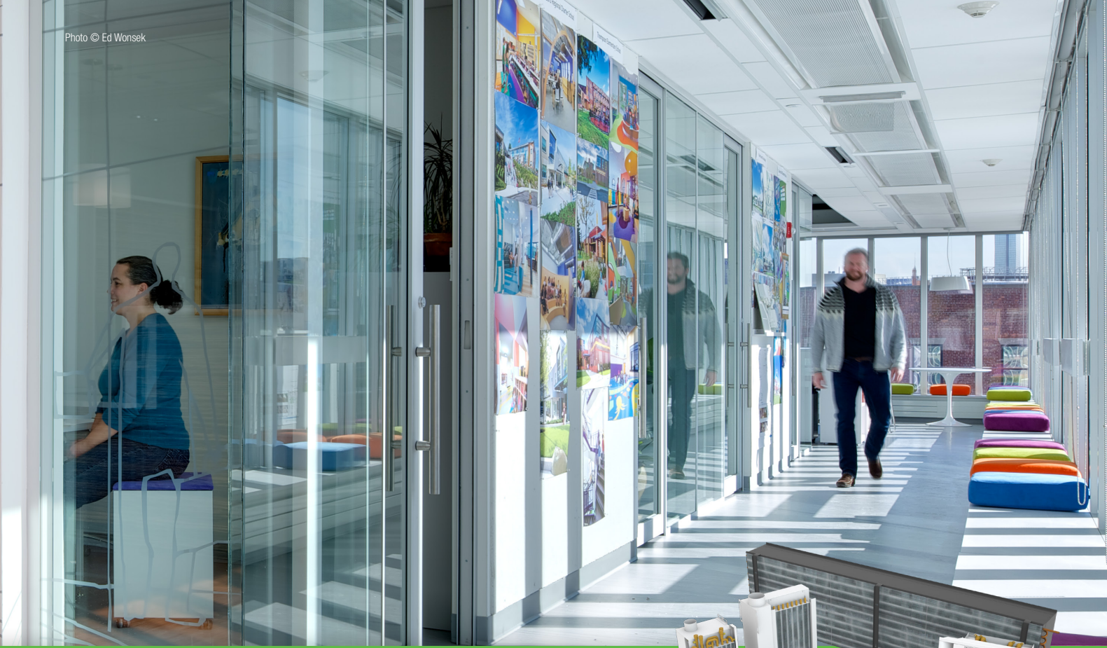
Above: Chilled Beams
